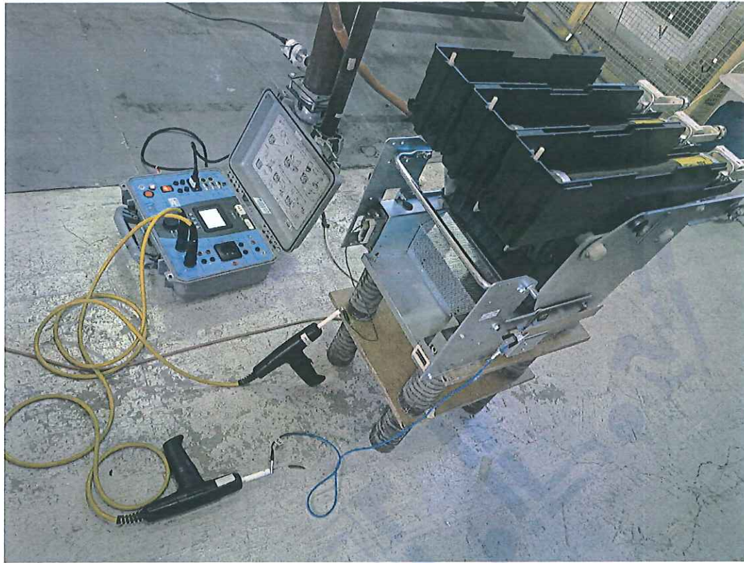
Figure 3: Equipment under dielectric test on auxiliary and control circuits
